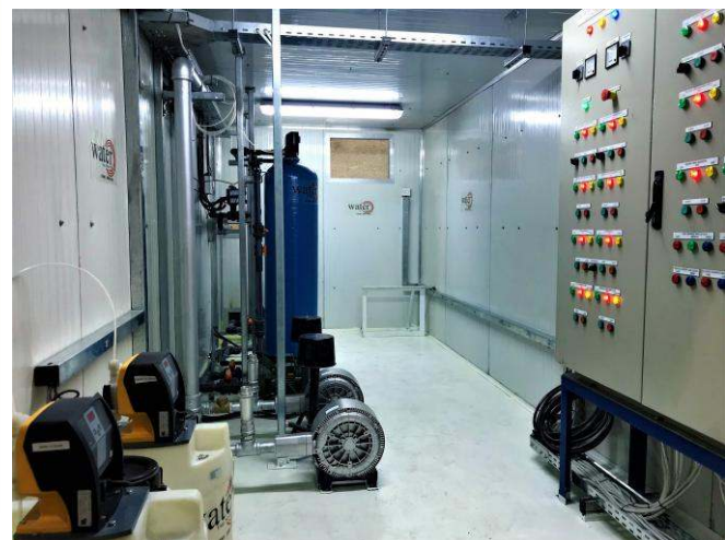
CONTAINERISED PLANT ROOM
