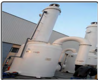
Chlorine Gas Scrubber
