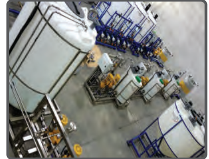
Chemical Injection Skid
