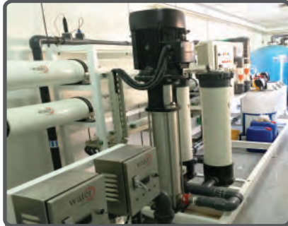
Reverse Osmosis System
