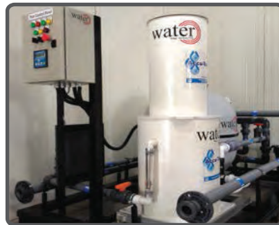
Swimming pool disinfection
