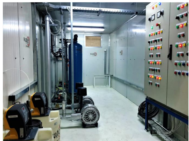
CONTAINERISED PLANT ROOM
