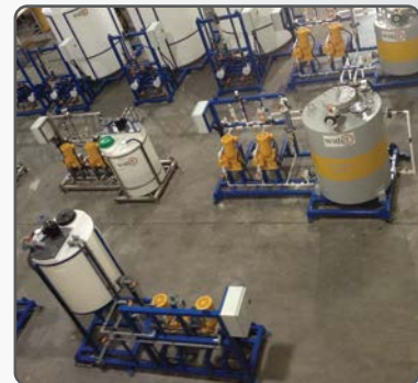
Chemical Injection Skid
