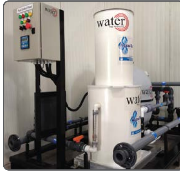
Swimming pool disinfection & Filtration system
