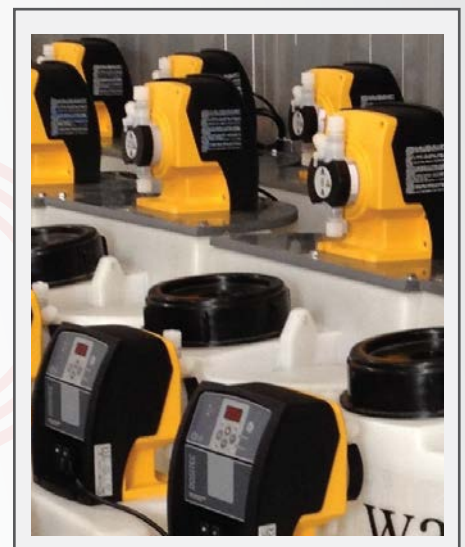
Dosing Pumps and chemical tank
