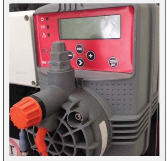
Pumps and chlorine and PH Probe and Housing
