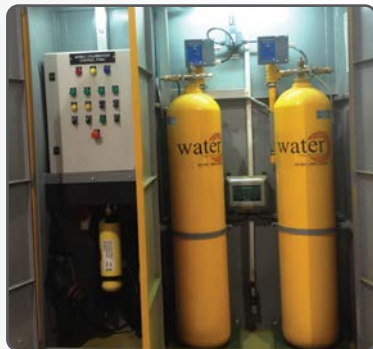
Gas Chlorination System
