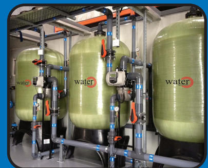
Containerised Water Treatment systems
