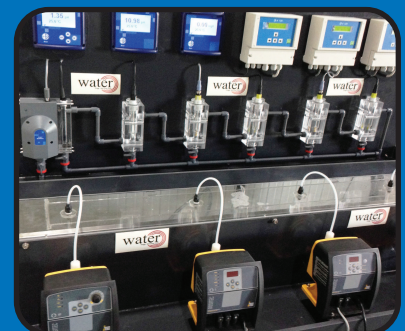
Water Quality Monitoring Systems cum dosing (WQMSD)
