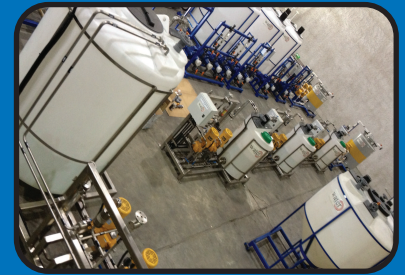
Chemical Injection skids
