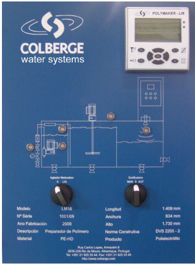
Process control panel of the preparer
